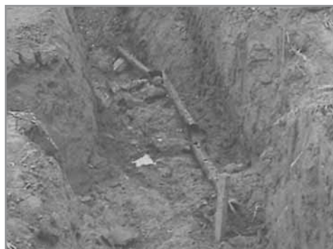
Figure 2.13 Exposed pipe mines lying in base of excavation (about 50 mm diameter pipe)
